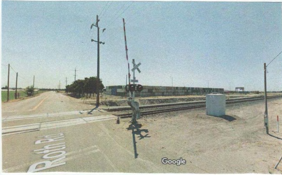
GRADE CROSSING SIGNALS AND GATE
