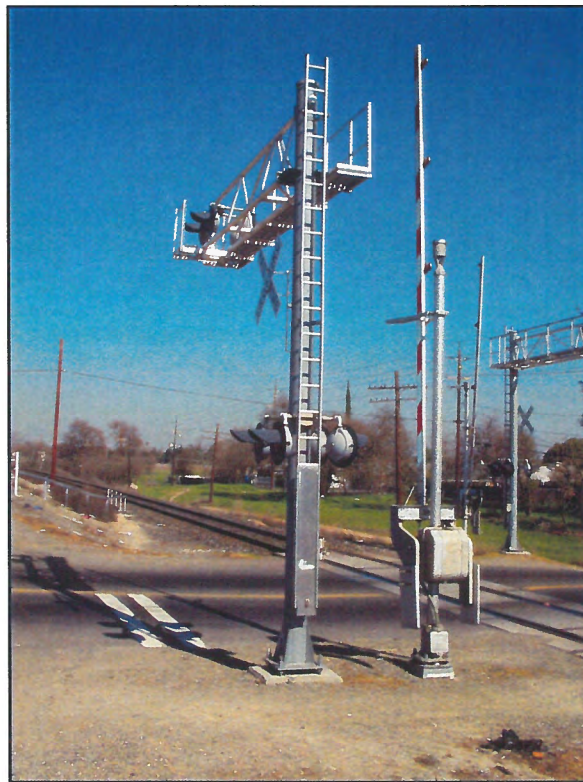
Modern crossing equipment at El Camino Avenue. View to northeast.
