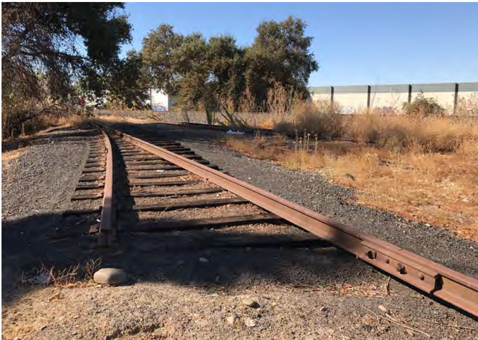
Photograph 4. Segment 2 of UPRR where two sidings split from the main line. Main line in background, sidings in middle and foreground, camera facing southwest, October 27, 2017
