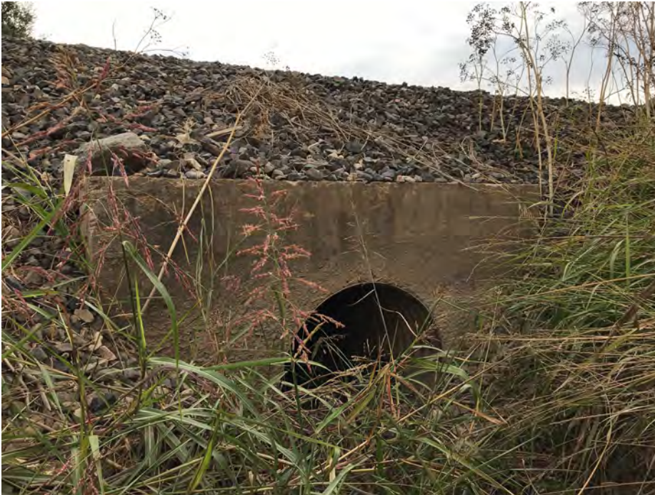
Photograph 2. Culvert under Segment 1 of WPRR, camera facing northwest, November 8, 2017
